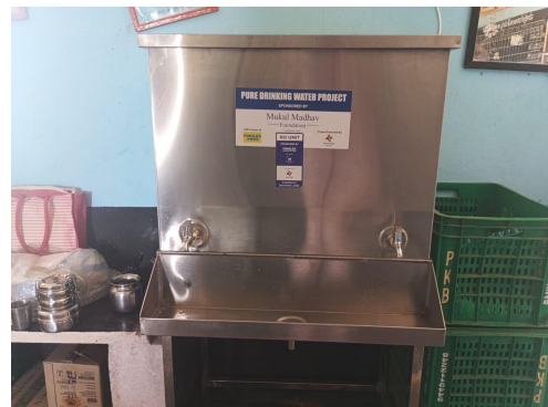
RO Purifier installed by Finolex for safe drinking water
